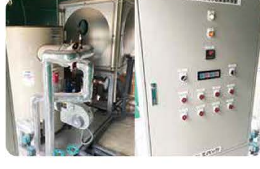
Boiler / Control System Stone Sauna Bed / Stone Sauna Room With carbon thermal sheets
